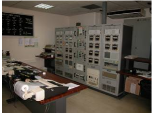
Riyadh Control Center
